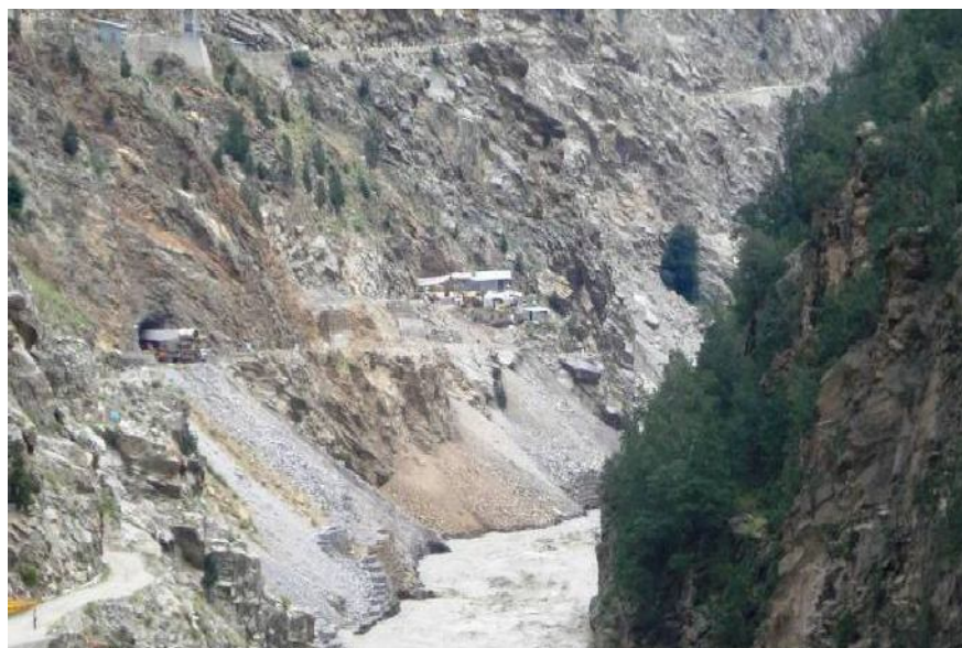
Photo-20: Construction work at power house site of Kashang stage-1- muck dumping sites are clearly not above HFL of Sutluj
