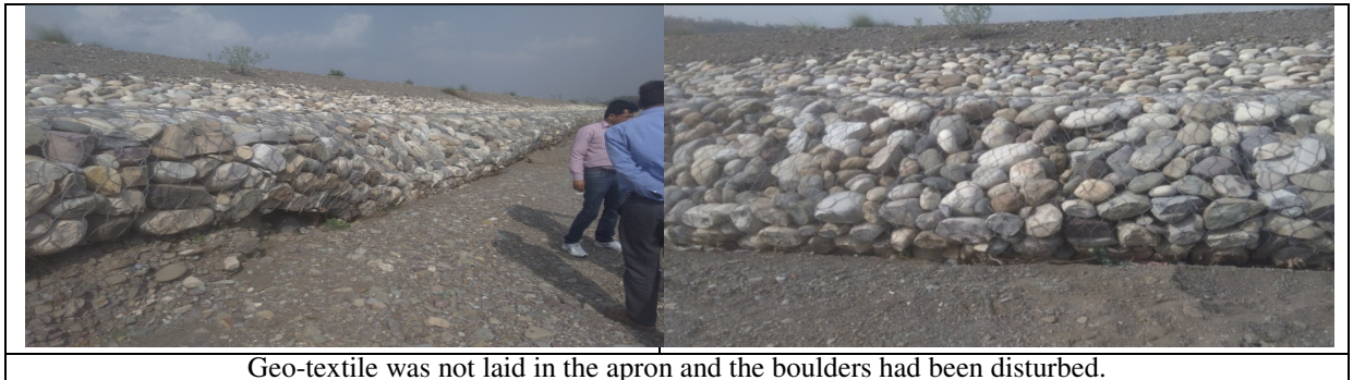
Geo-textile was not laid in the apron and the boulders had been disturbed.
